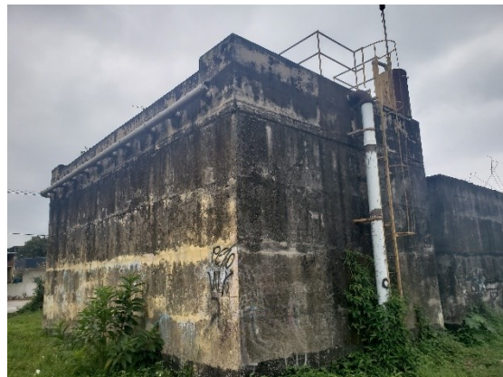
FIGURA 6-54 – ETE FRADE – REATOR UASB
