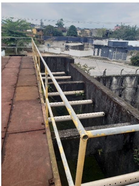
FIGURA 6-55 – ETE FRADE – REATOR UASB – VISTA SUPERIOR
