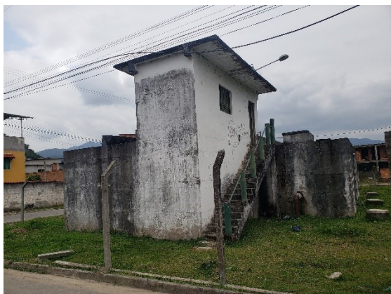
FIGURA 6-12 – ETE FRANCISCO GUEDES – VISTA GERAL
