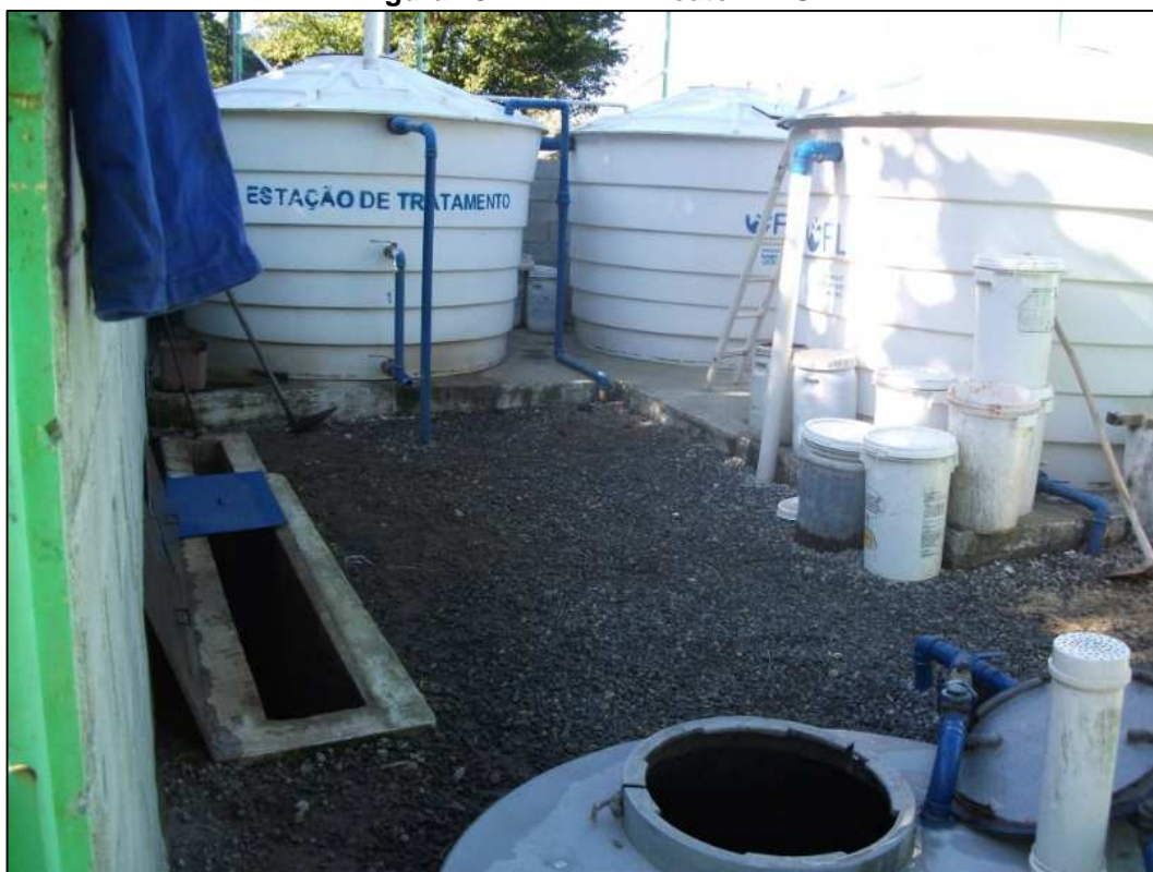
Figura 28.71 – ETE – Reator RAC
